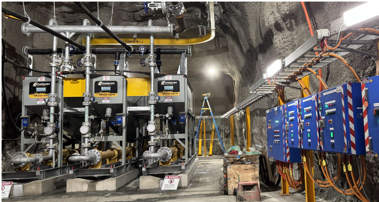
Figure 4 – Three WT107 pumps in 801 level
