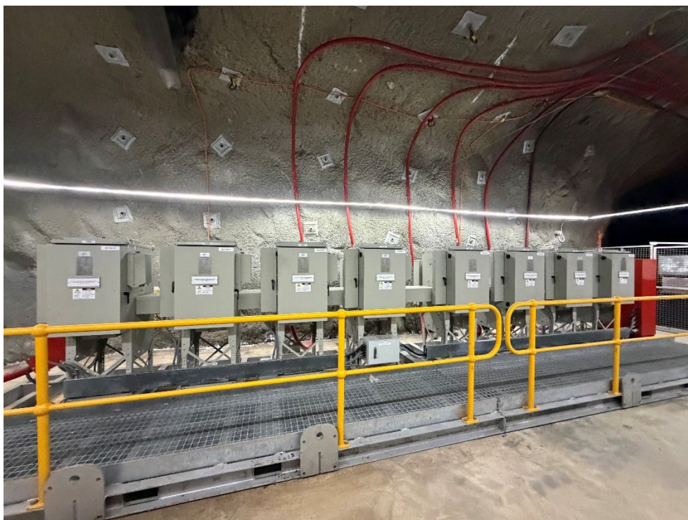
Figure 6 - Ring main unit linking newly installed redundant power cable to underground power network
