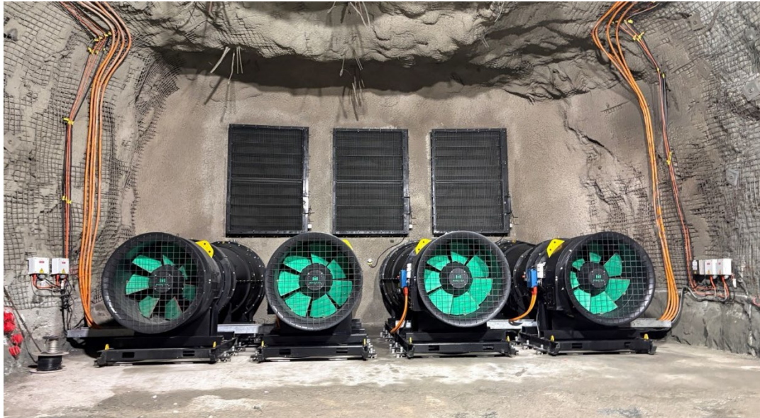
Figure 2 – Installed Interim fans
