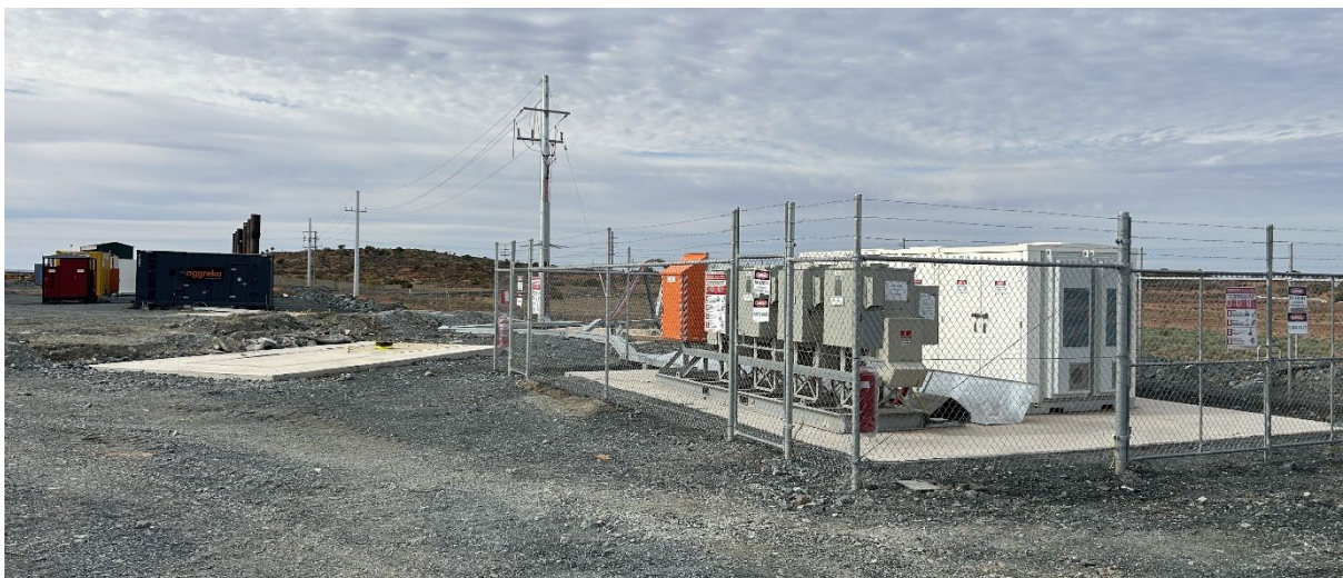
Figure 5 – Newly installed surface power infrastructure for Beta Hunt
