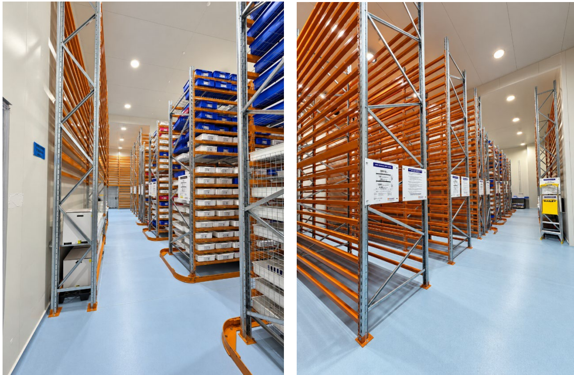
Figures 1 and 2 Racking installed in the extended 2°C to 8°C cool room at South Granville
