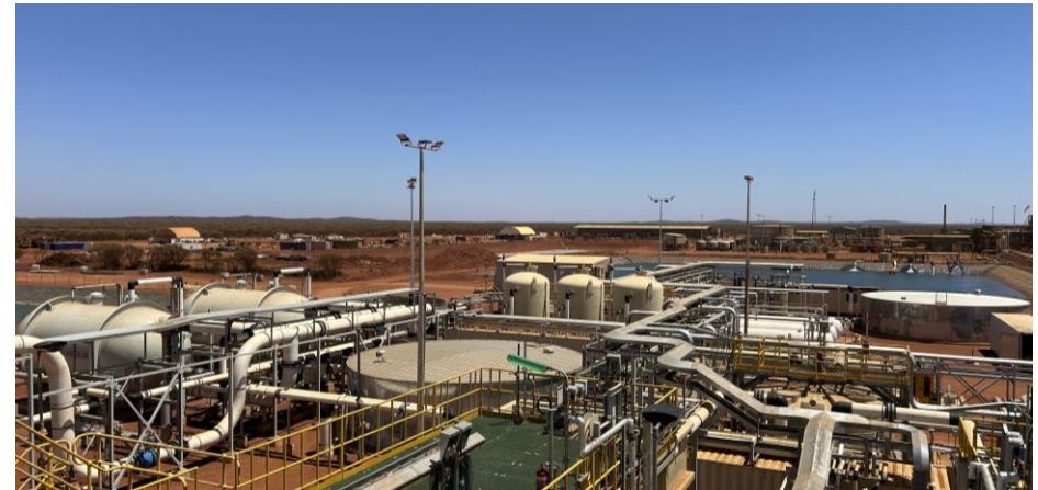
Mt Weld Recycled Water Treatment Plant
