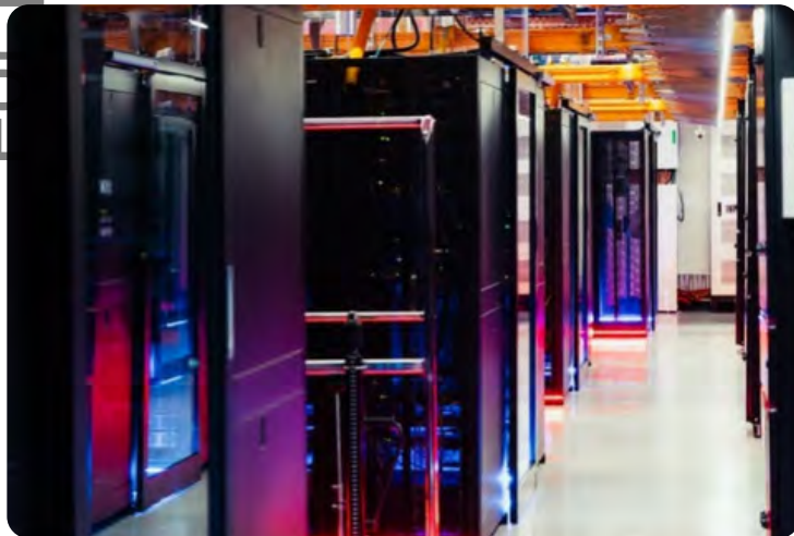
Datacentre220 – our first Express Connect installation
