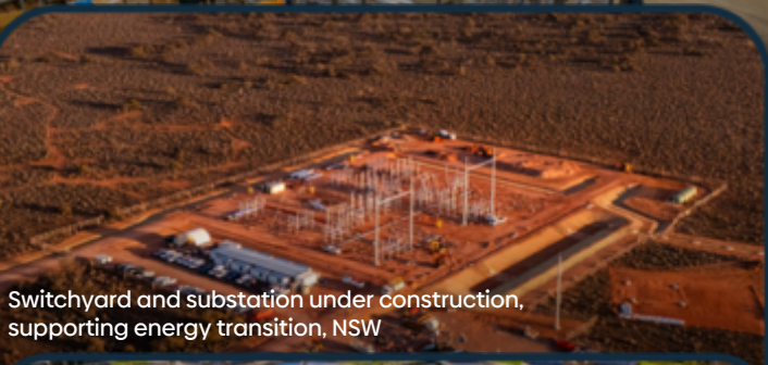
Our in house switchboard manufacturing capability supporting the energy transition, NSW
