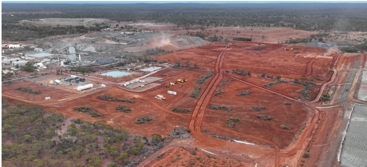
Figure 1 - Drone View showing earthworks commenced for new 3.0Mtpa Processing Facility (looking NW)
