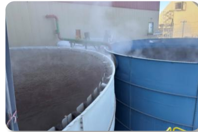
Thickener and process water tanks
