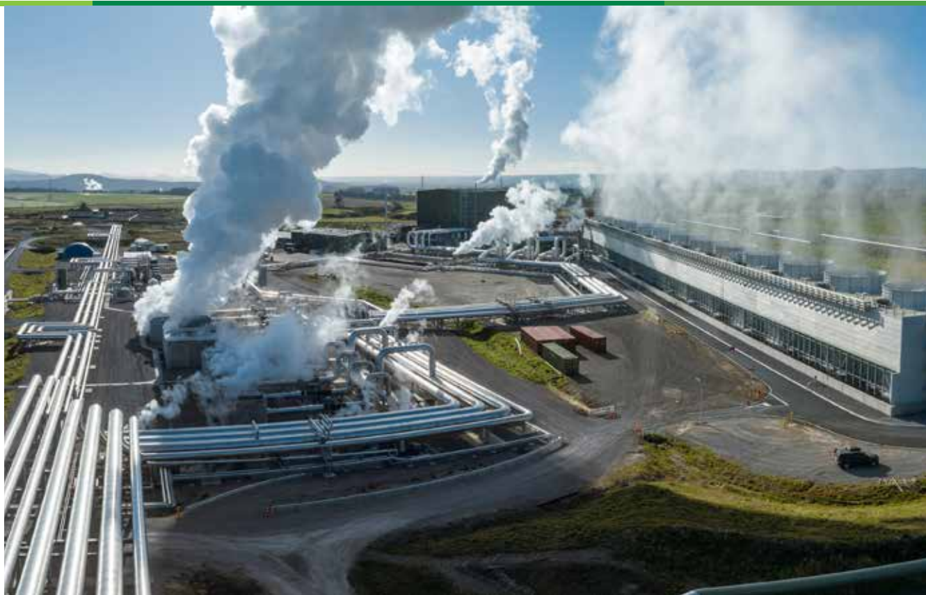
Contact's geothermal steam turbine power station at Tauhara, in Taupō, New Zealand.
