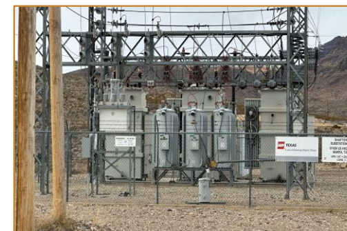
Shafter Electrical Infrastructure
