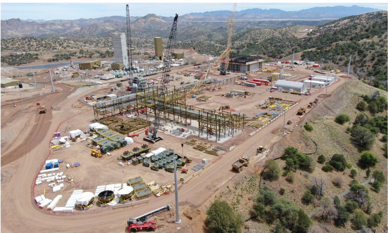
Figure 2: Hermosa surface infrastructure as at April 2026
