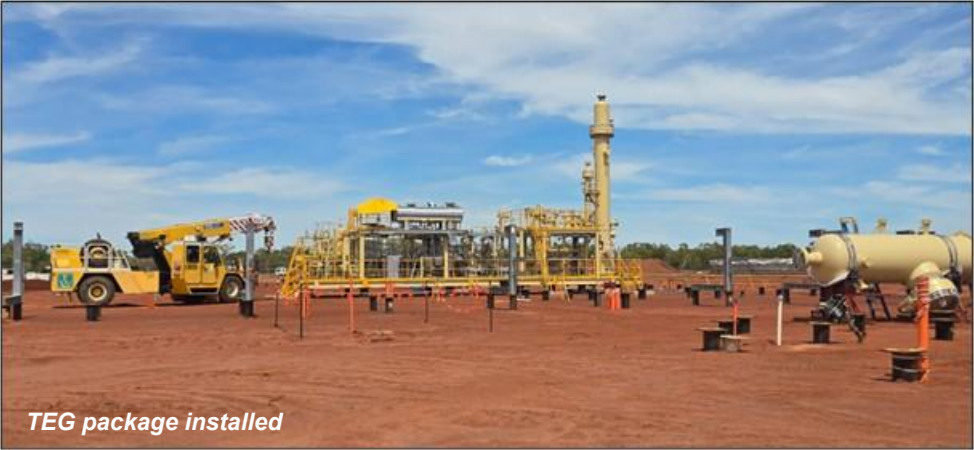
Compressor units installed on SS2 pad
