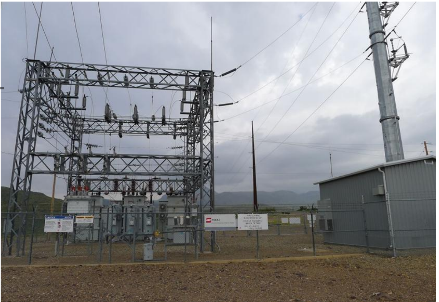
Figure 7: Shafter Mine and Processing Substation.
