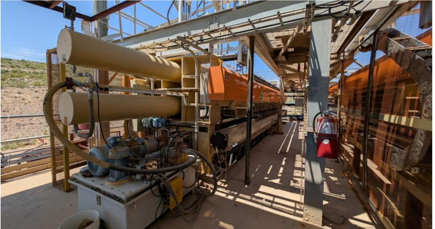
Figure 6: Shafter Processing Facility Filter Press (one of two filter press')
