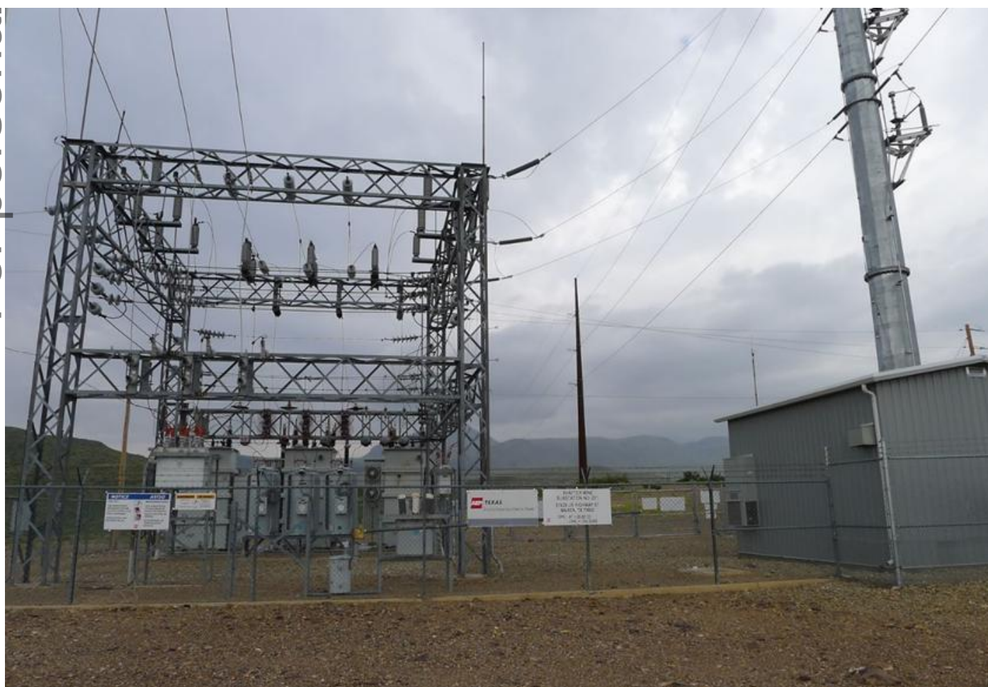
Figure 5: Shafter Mine and Processing Substation.
