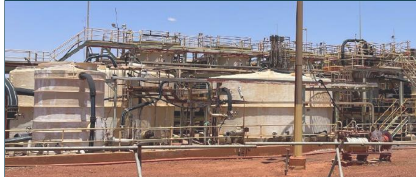
SX Plant (“Solvent Extraction”) requires new pumps, motors, electrical and controls
