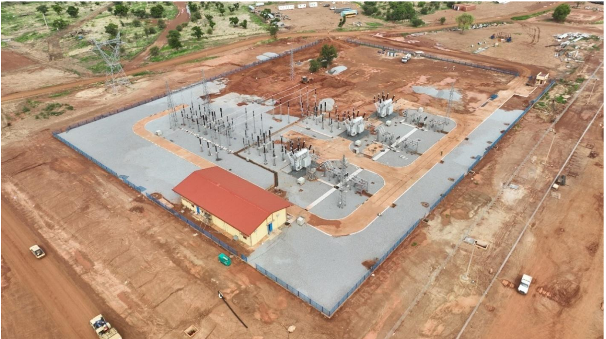
Kiaka Electric Power Substation
