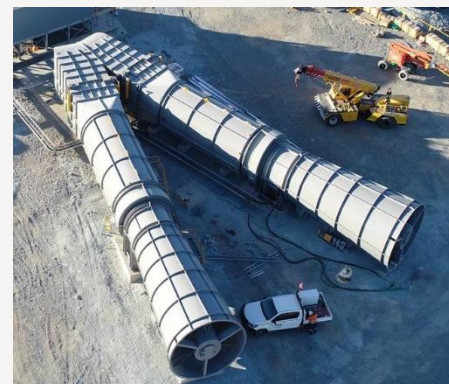
Underground primary ventilation
