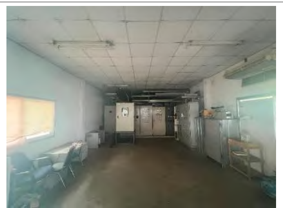
Internal view of the single-storey water chiller control building
