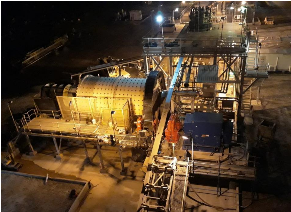
Figure A13: Existing 1800kW Ball Mill
