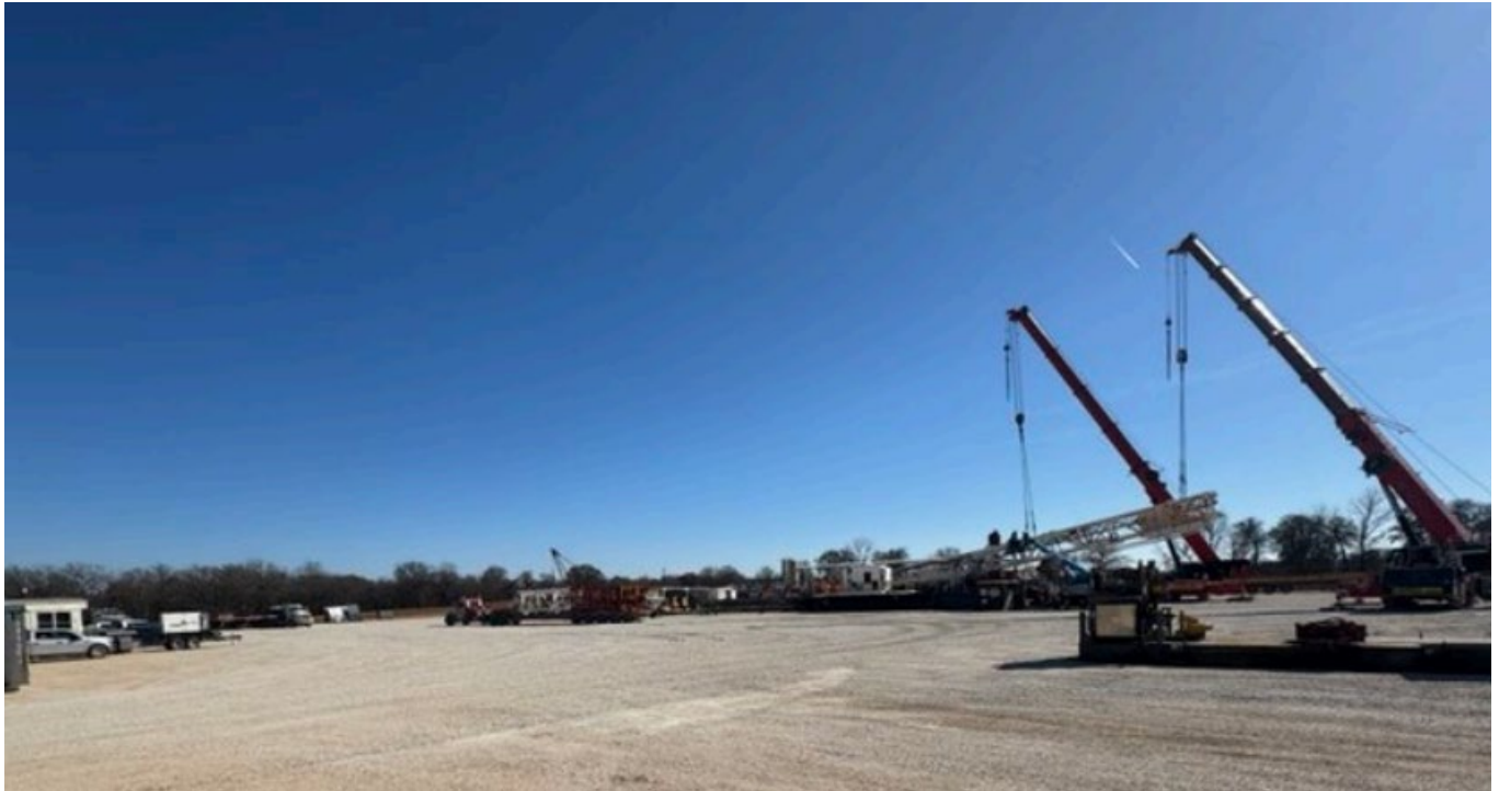
Figure 5: Rigging up Kenai Rig 19 on the Bruins pad in Carter County, Oklahoma.
