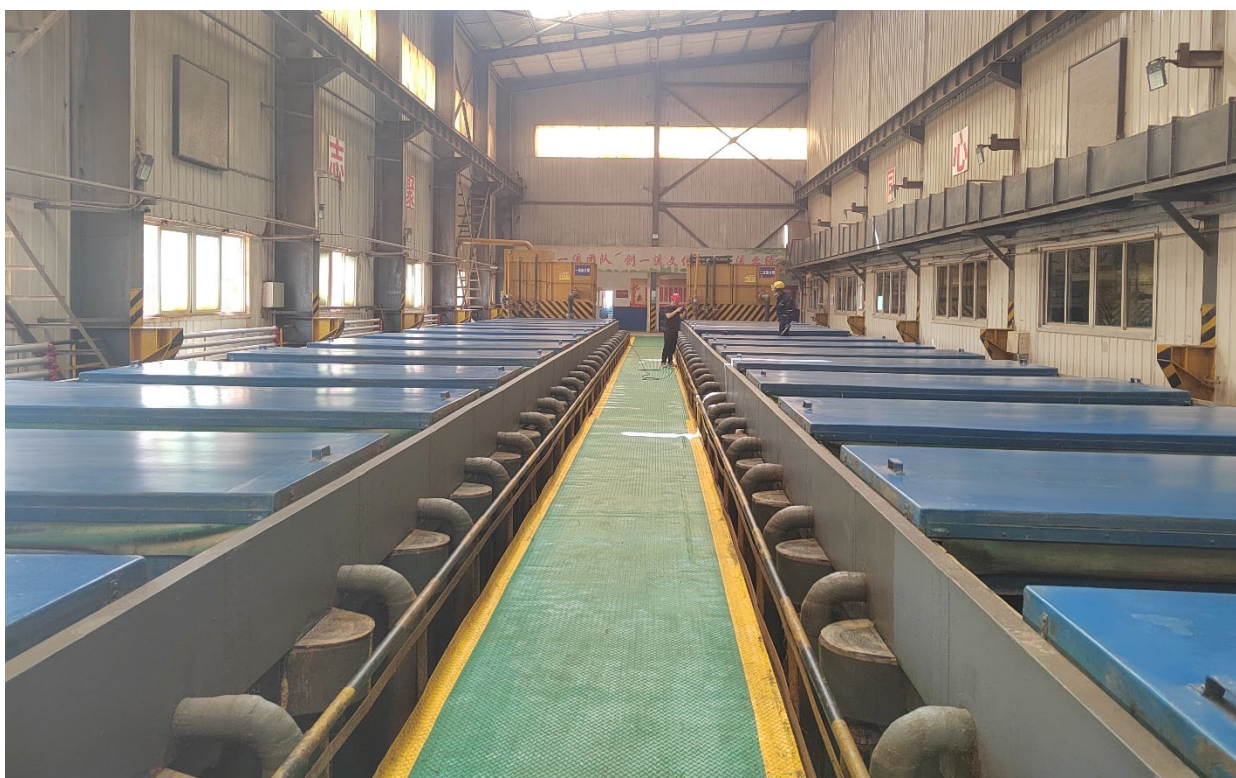
4,000tpa Antimony Electrowinning Circuit installed by BGRIMM Technology, Gansu Zhaojun, China
