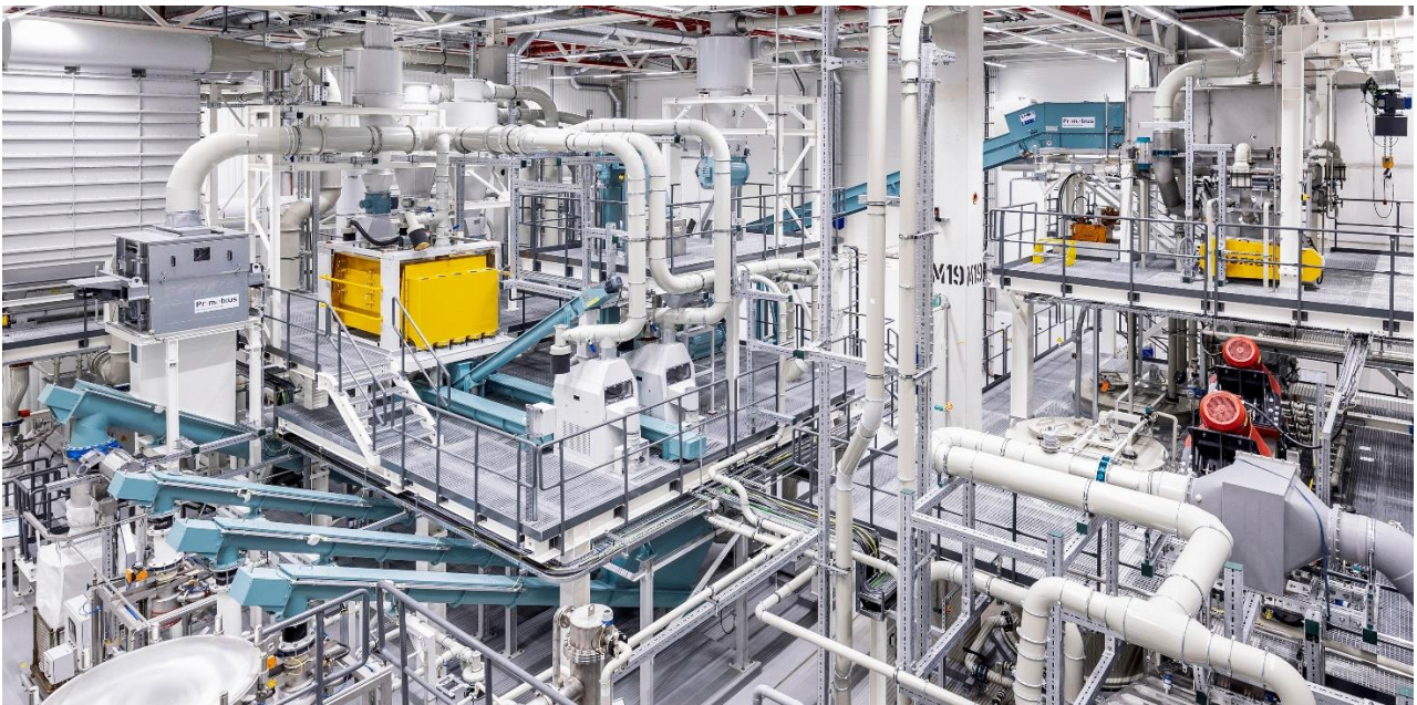
Figure 1 – Part of the Integrated LiB Plant installed by Primobius at Kuppenheim
