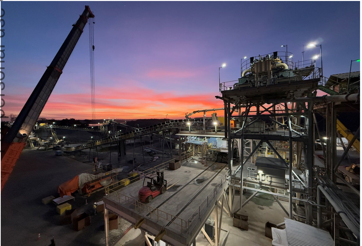
Figure 2 | Okvau Gold Mine Processing Plant
