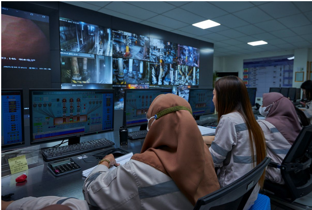
Nickel Industries' RKEF operations control room
