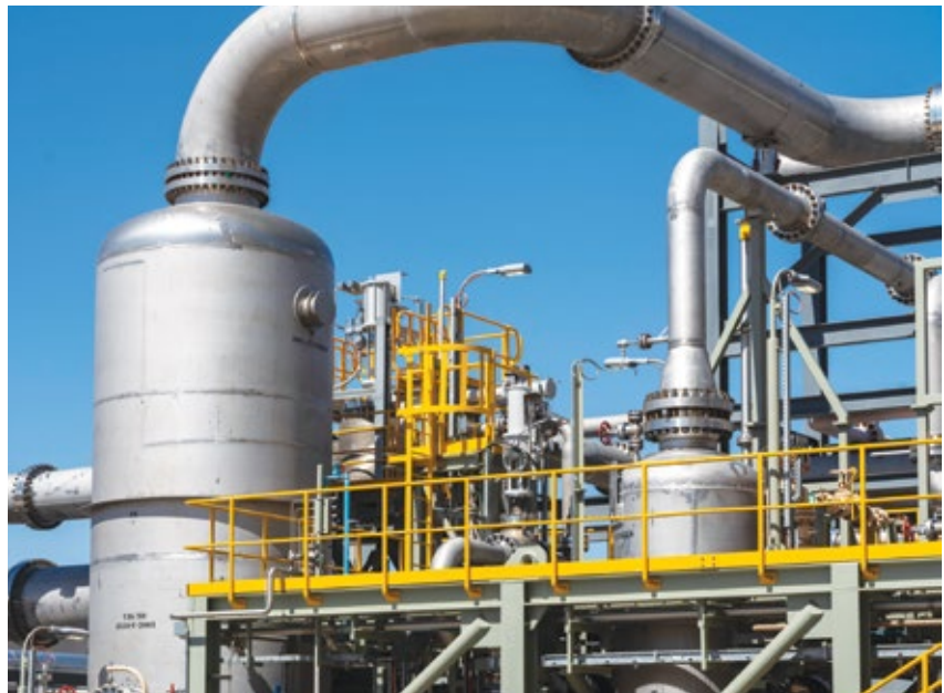
Pictured: The Moomba CCS facility
