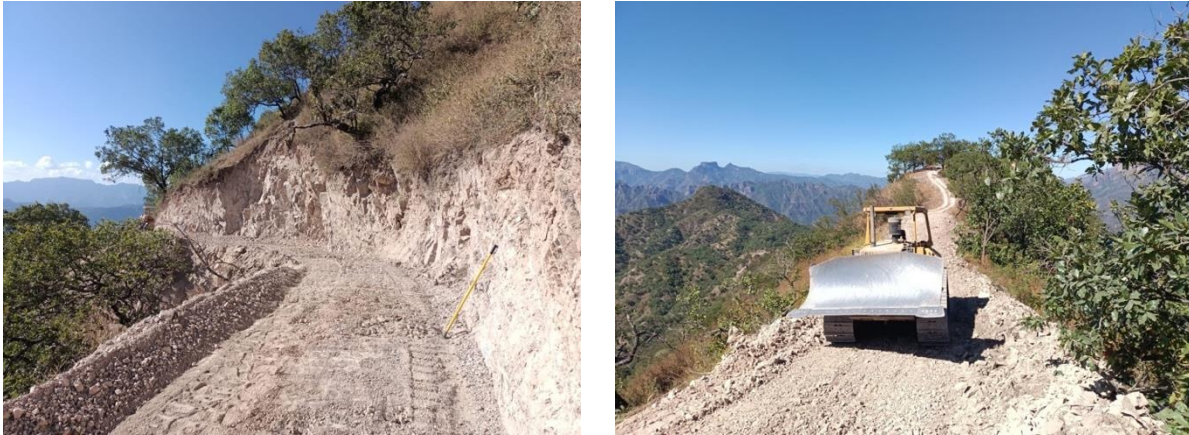
Figure 75 left and right - municipal road upgrade works, facilitating the expanded exploration program for the Copalquin District in 2025
