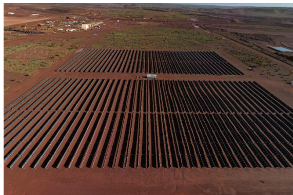
Solar array at Ken's Bore
