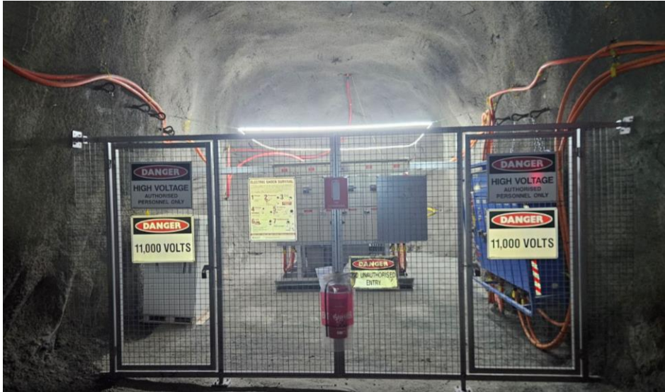
Figure 14 - Underground electrical sub-station
