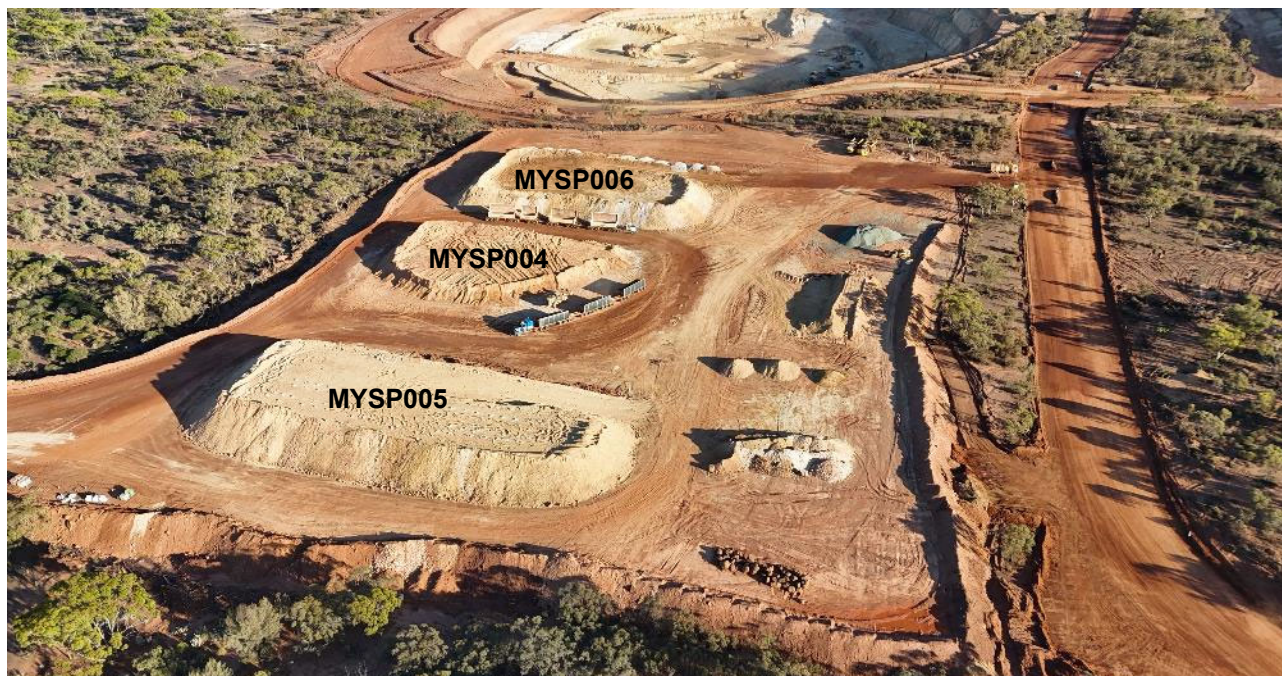
Figure 1: Myhree ROM pad (looking north) showing current stockpiles being hauled or under construction
