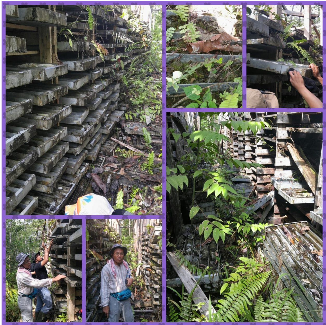
Photo 2. Condition of Tekai Coreshed on 2 November 2016
