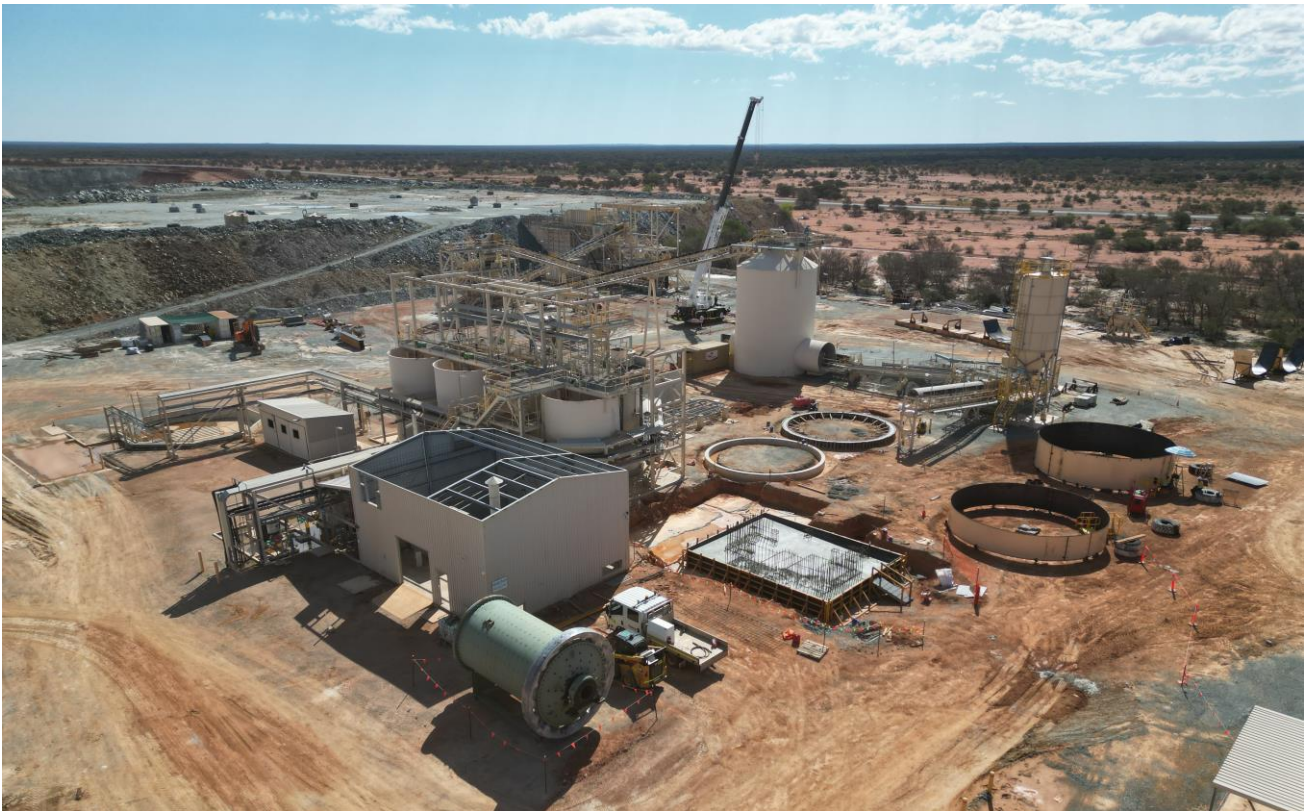
Figure 40 – View of expanded grinding area and ball mill plinths with new larger 750kW ball mill positioned ready for installation (November 2024).
