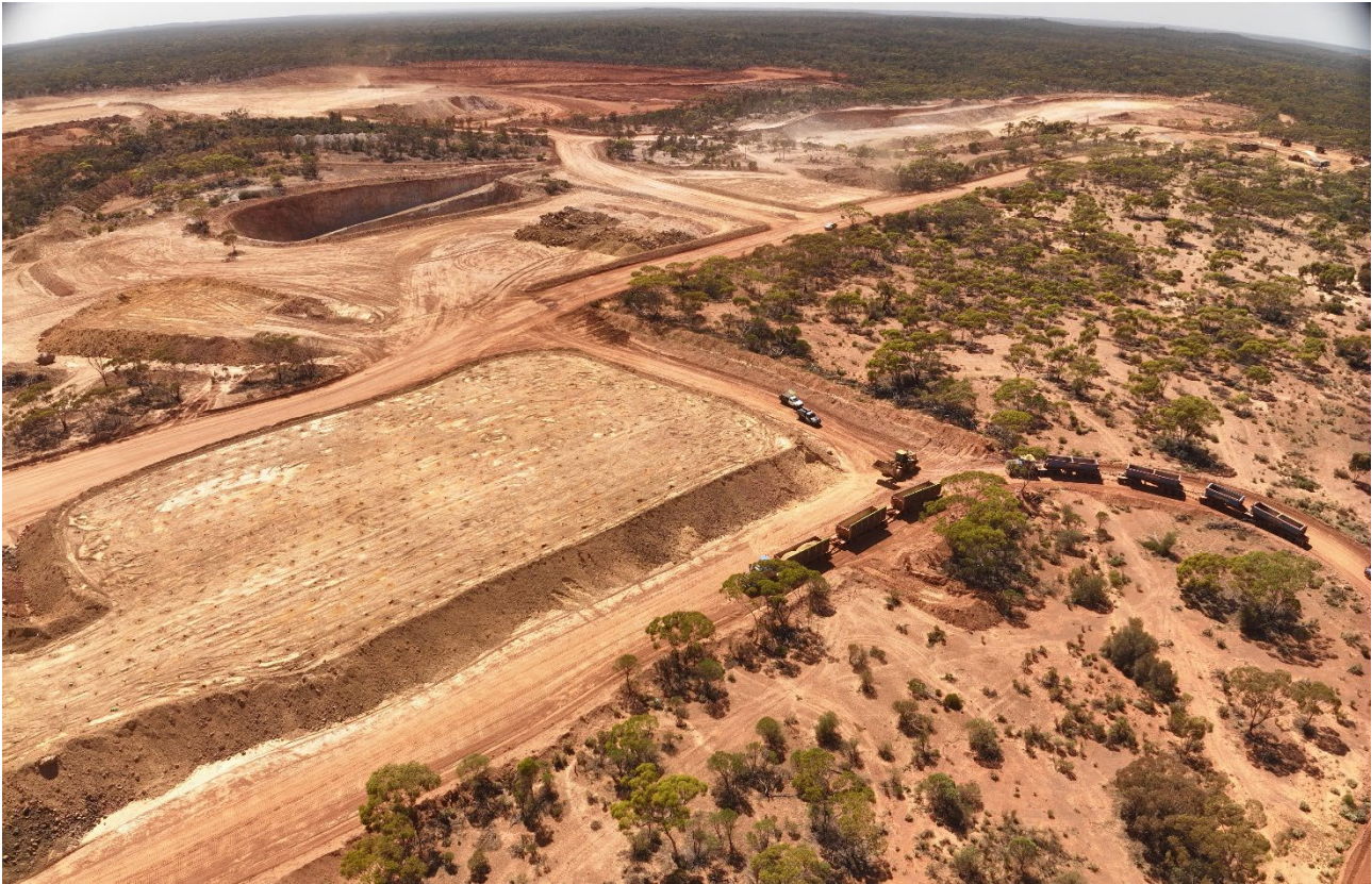
Figure 2: First road trains loading ore with open pit operations in the background
