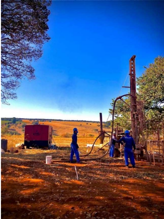
Figure 6: Reverse circulation drill rig in the backdrop of vast pastureland of CODA North.
