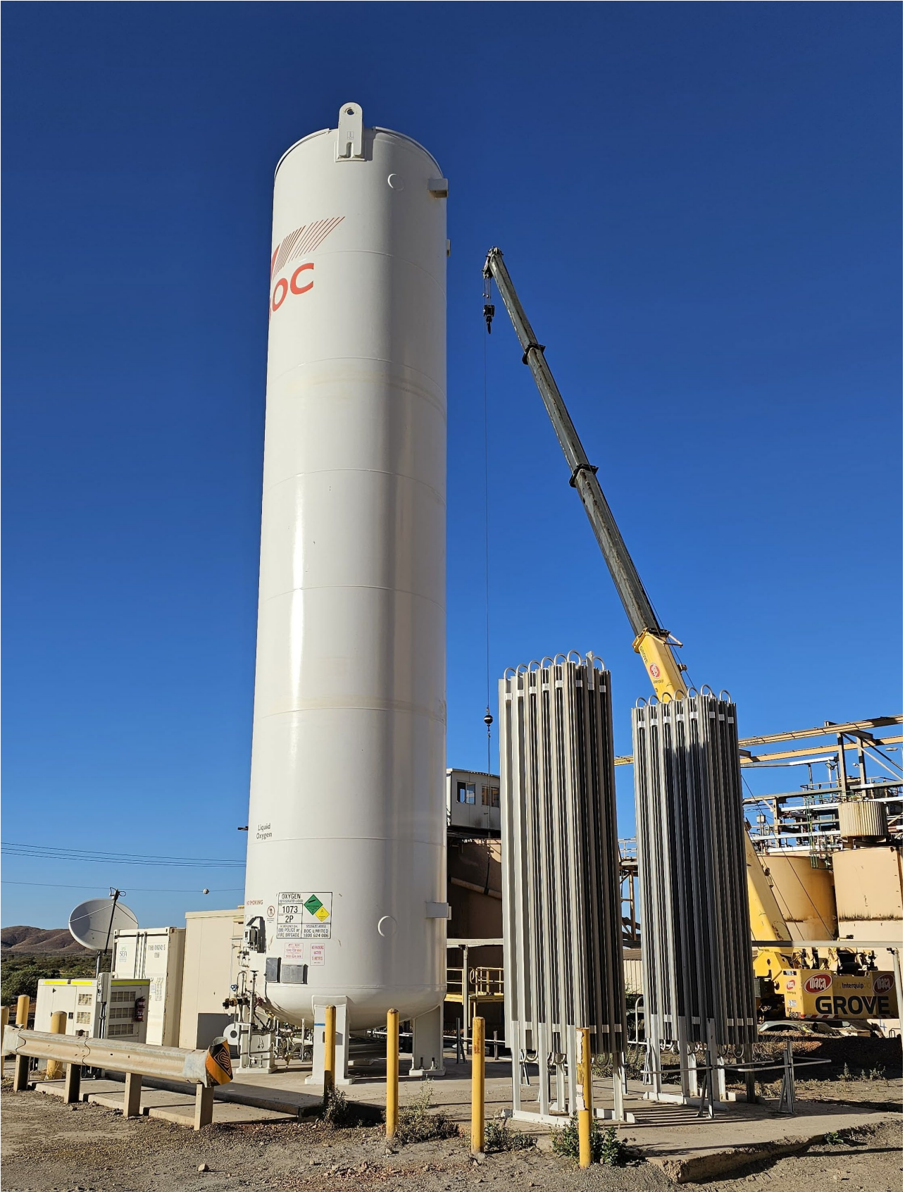
Figure 5: Showing the newly installed oxygen storage tank.
