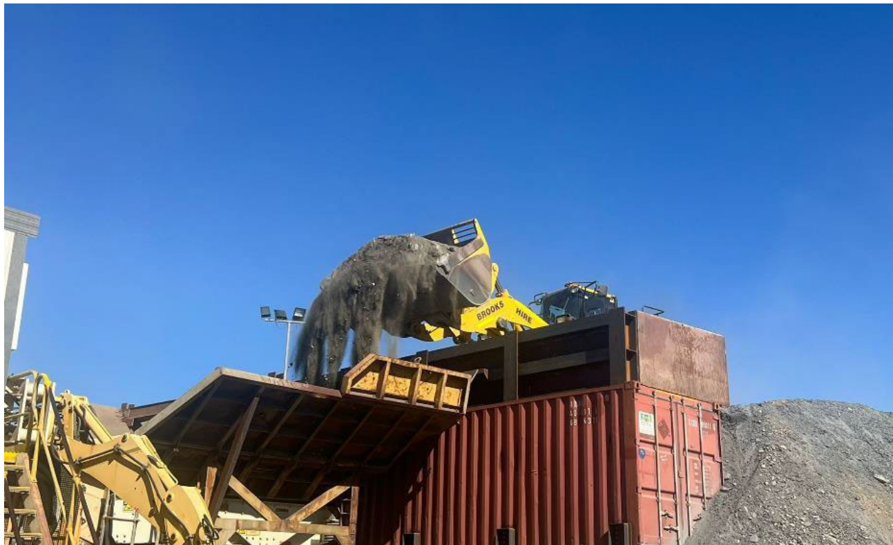
Figure 1: Crushing underway – low-grade commissioning Ore being tipped into crushing circuit as wet commissioning commences.
