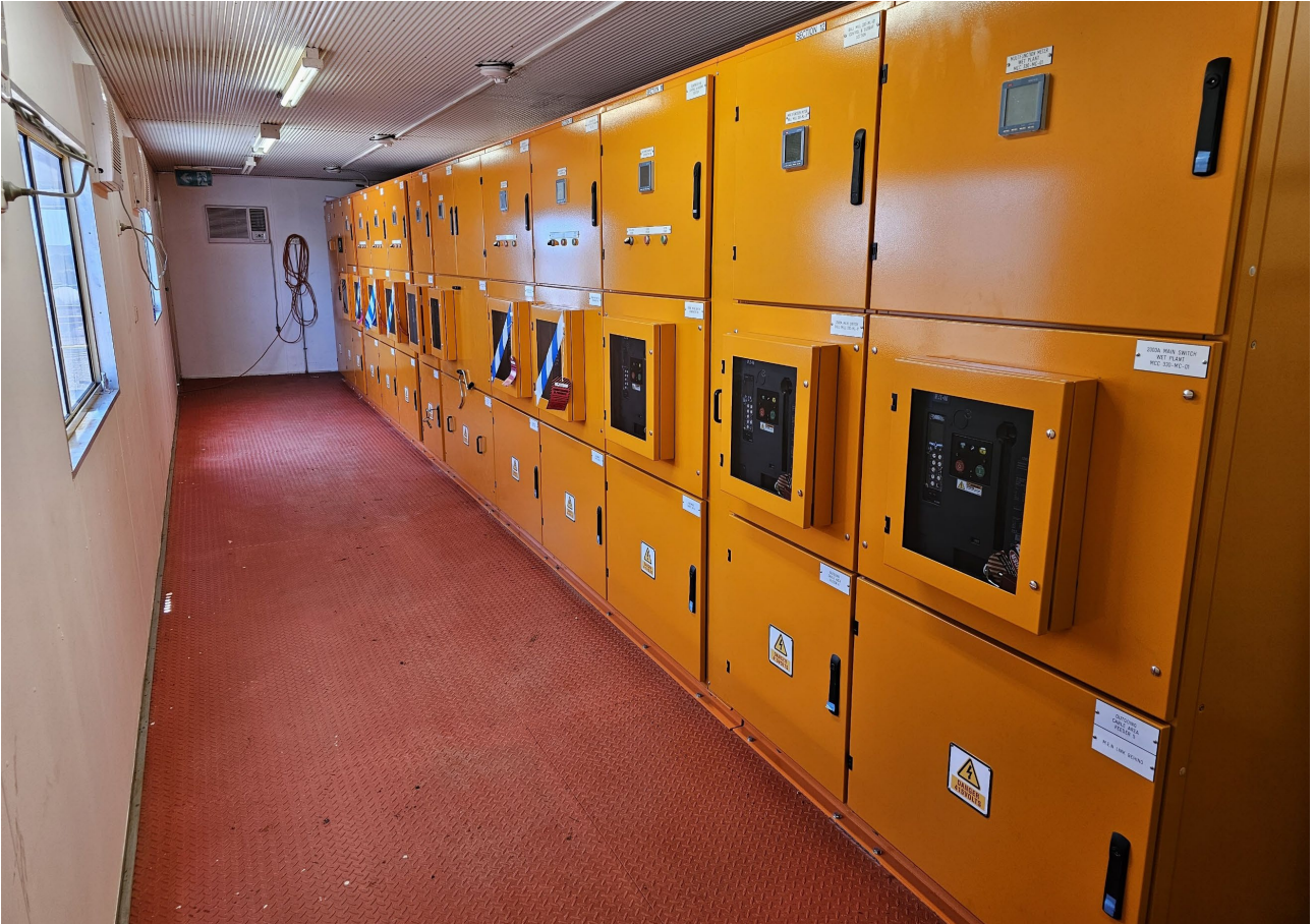
Figure 3: Showing the newly installed 415-volt switchboard at power station # 1.
