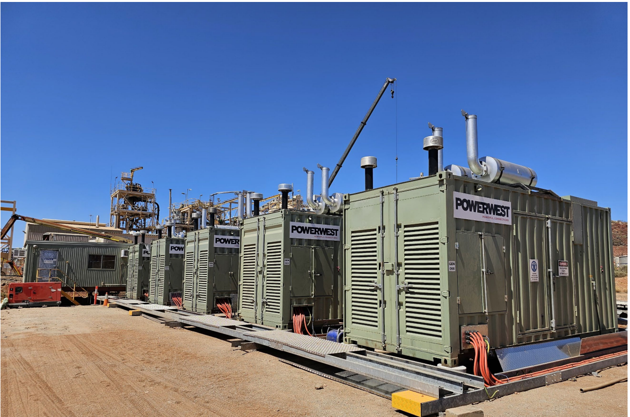
Figure 4: Showing the 5 x 880 KVA generators installed at power station # 1.
