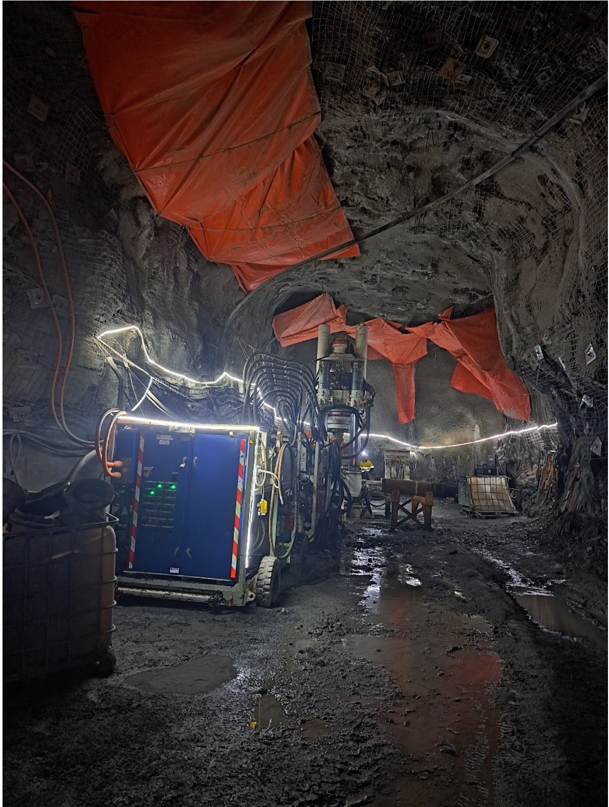
Figure 5 - Long-term ventilation infrastructure under development.
