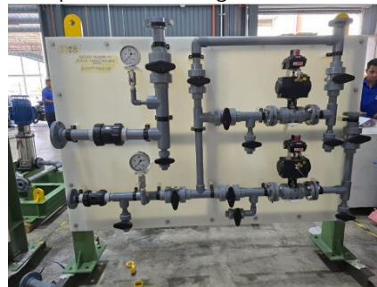
Filtrate Receiver to Storage Tank Piping
