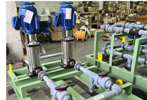
Cloth Wash Pumps Skid
