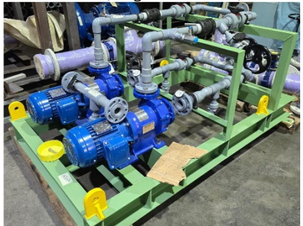
Filtrate Return Pumps Skid
