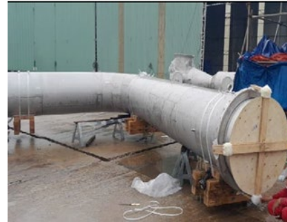
Main Ducting to Venturi Scrubber
