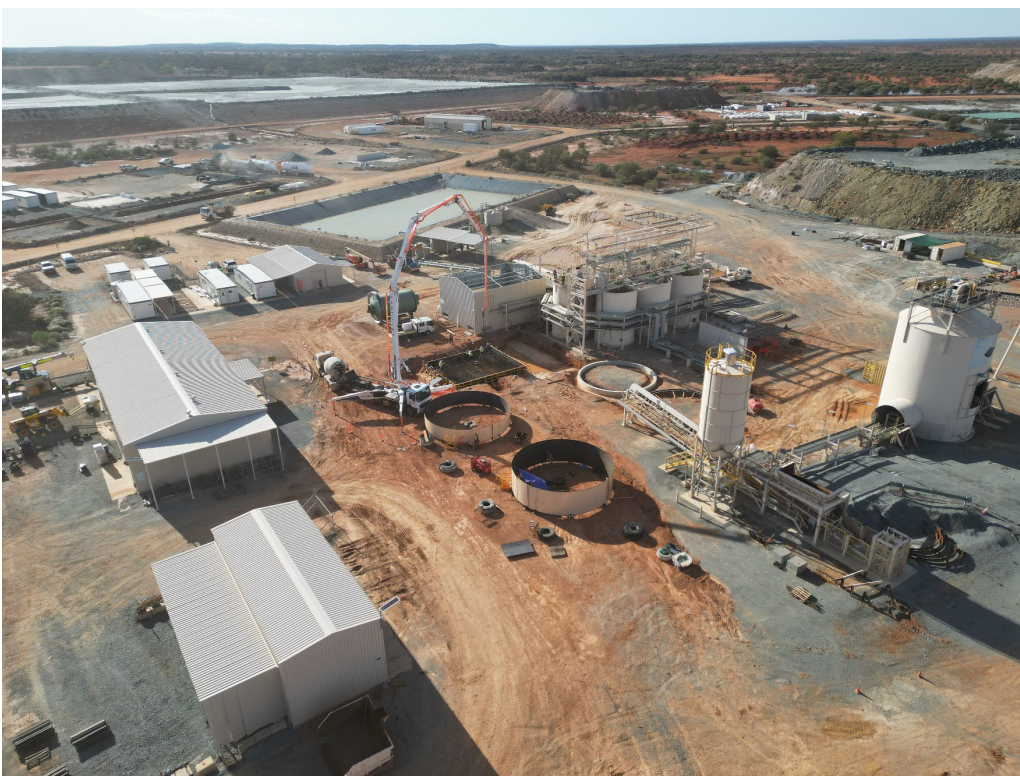
Figure 2: Drone image of ball mill foundation works and ongoing tank skin fabrication, November 2024.
