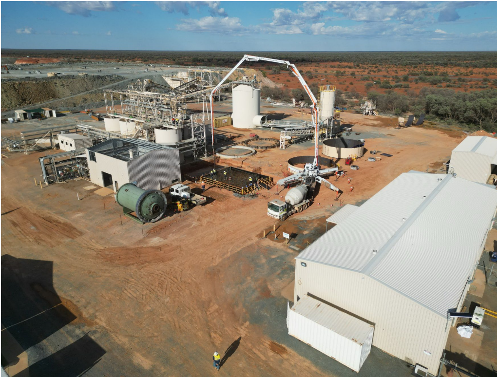
Figure 1: Drone image of concrete pour for ball mill foundation in the foreground and ongoing tank skin fabrication visible in the background behind the concrete pump, November 2024.
