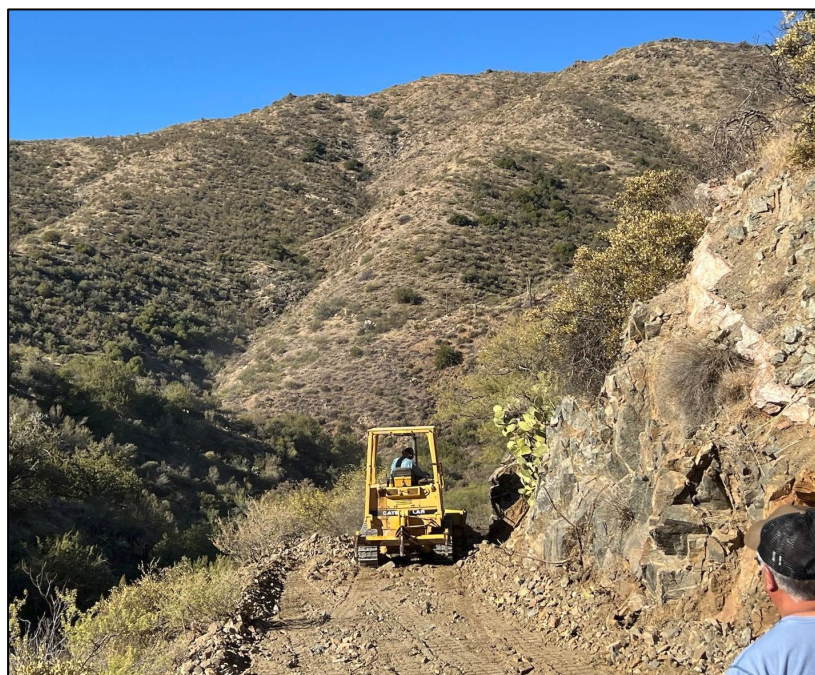
Photo 1 – Earthworks in progress to establish drill pads aimed at testing porphyry-style targets.
