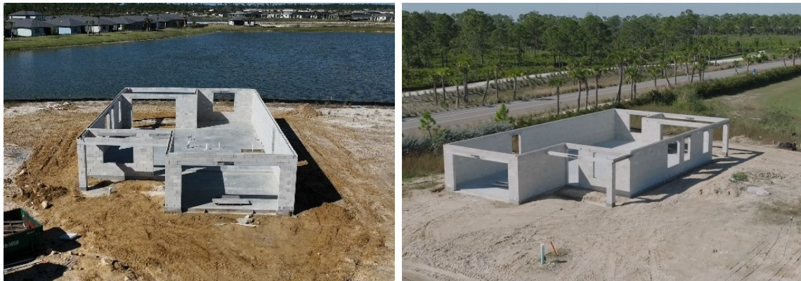
Recently completed houses seven (left) and eight (right) of 10 home Demonstration Program
