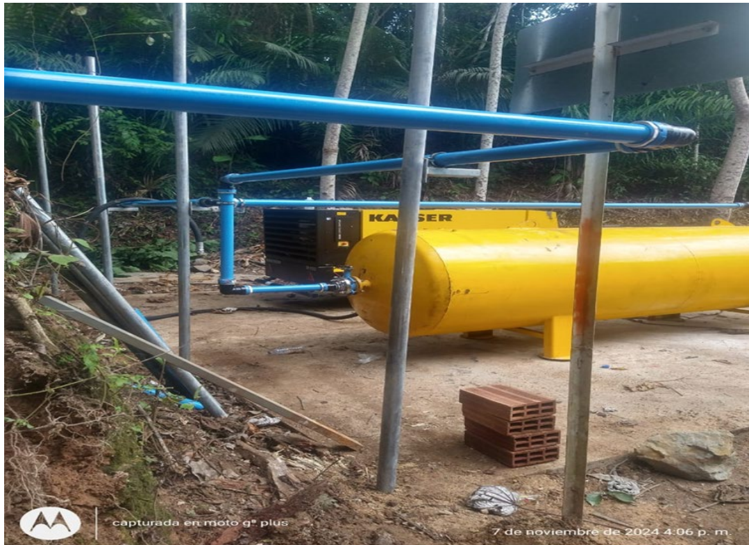
FIGURE 2: NEWLY INSTALLED COMPRESSED AIR SYSTEM FOR UNDERGROUND PRODUCTION DRILLING
