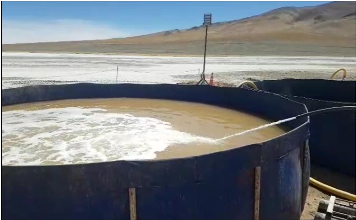
Figure 3. 10,000 litre tank being filled from brines during the 3 day pump test.
