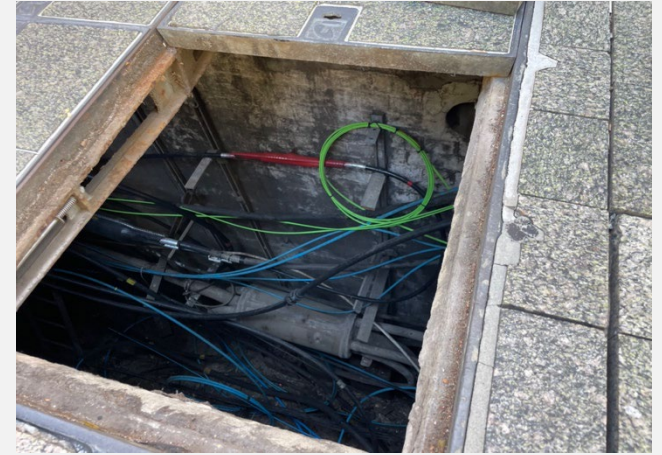
Protection of communication pits
