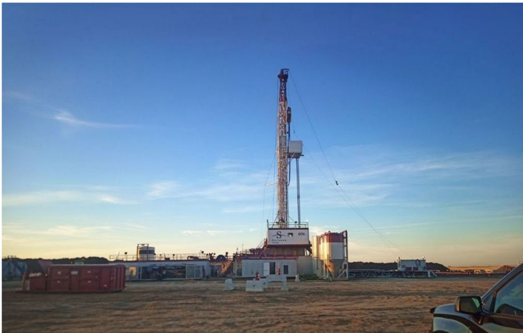
Figure 8: Drilling Well #3 on Pad #1. Well #1 and Well #2 can be seen in the foreground of the drilling rig
