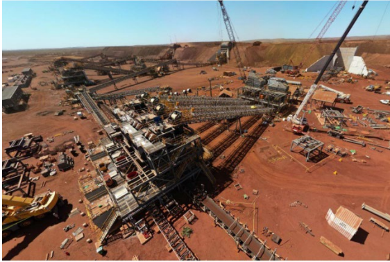
Three crushing trains at Ken's Bore
