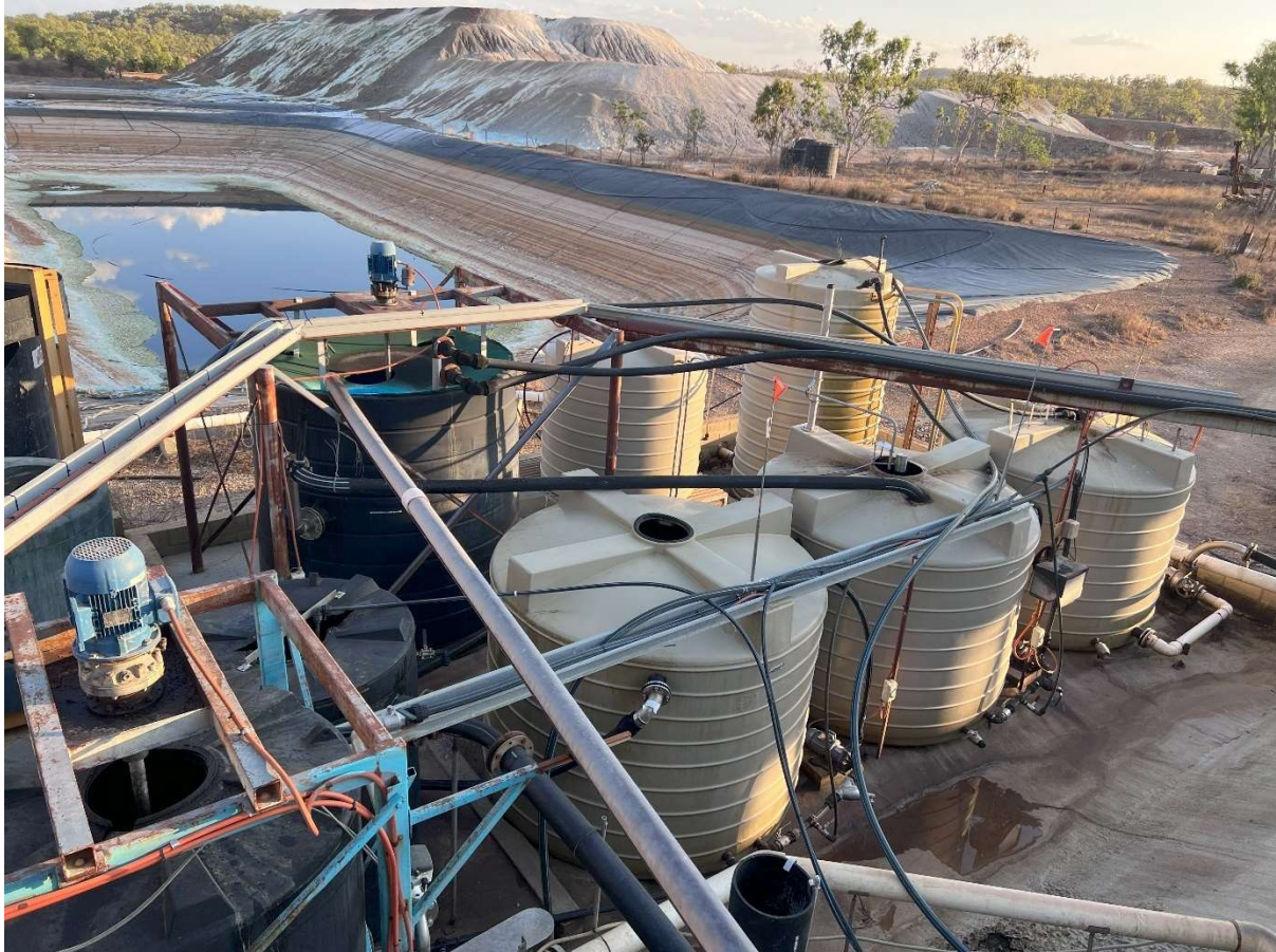
Figure 5. Picture of the SX plant, heap leach pads and liquor ponds at Tartana Plant
