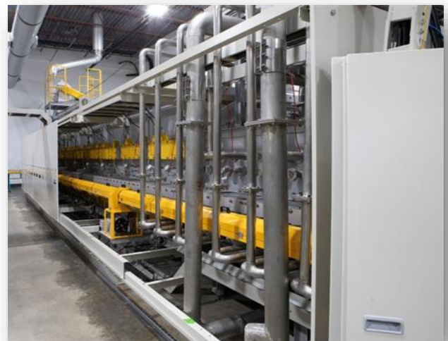
Figure 4 NOVONIX Cathode Pilot Line, Nova Scotia, Canada. 13.5 m long roller hearth kiln (RHK)
