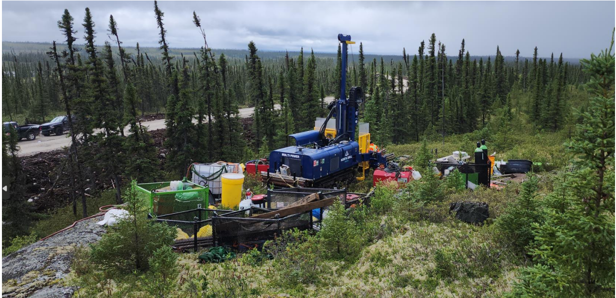
Figure 8: Geotechnical hole CV24-570 situated north of CV5 at a proposed infrastructure site.
