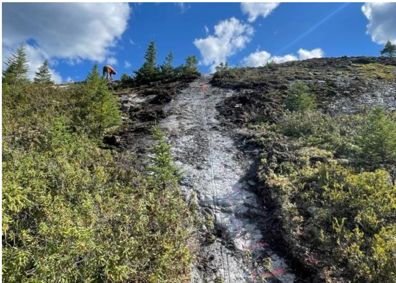
Figure 15: Saw-cut channel ready for sample layout marking at the CV5 Spodumene Pegmatite.
