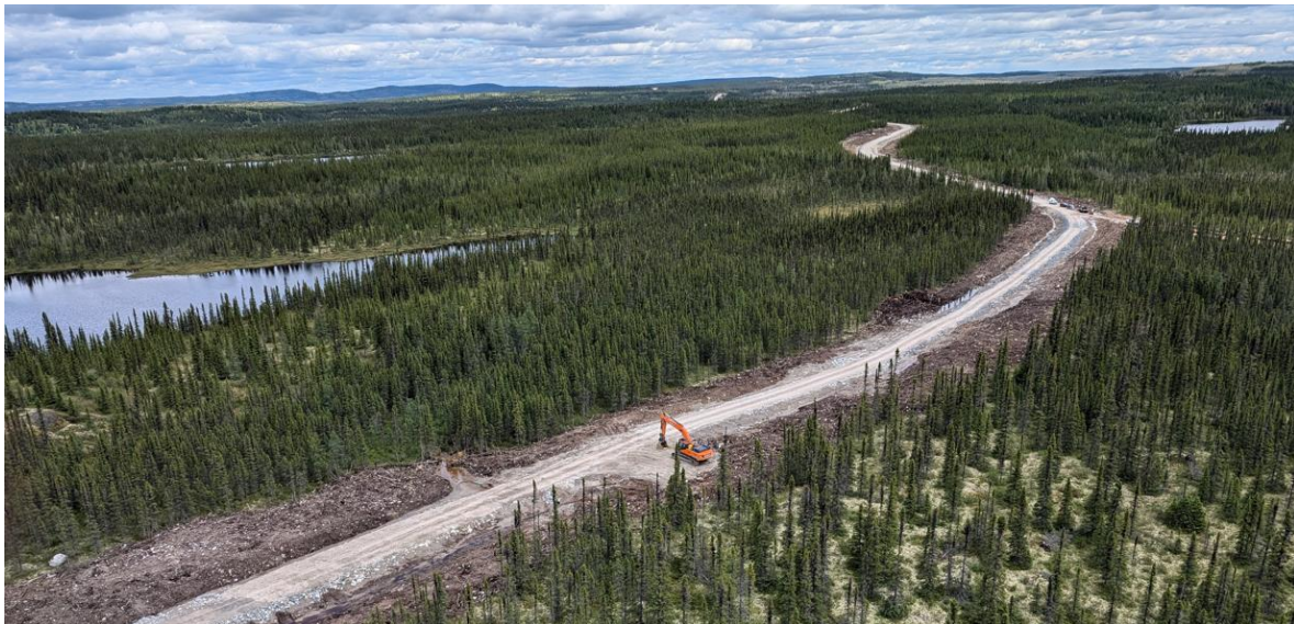
Figure 2: The Company's all-season road, extending south from the all-season Trans-Taiga Road, provides direct ground access for drill rigs to the CV5 Spodumene Pegmatite.
