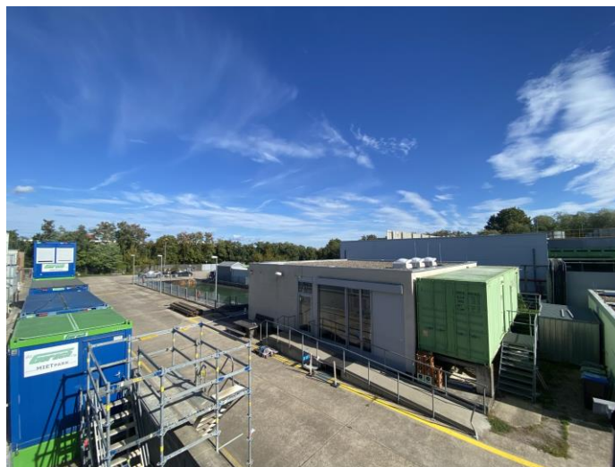
Figure 3 Geox geothermal power plant in the City of Landau.
