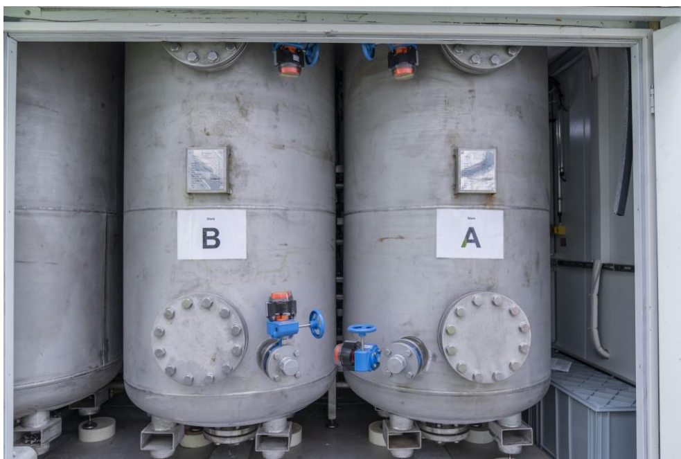
Figure 2 A-DLE unit at Vulcan's downstream lithium optimisation plant.
