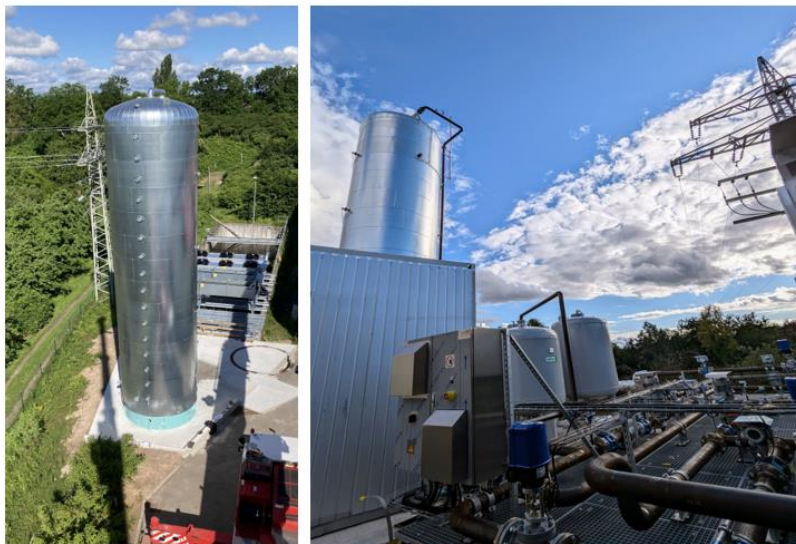
Figure 1 Thermal energy storage system installed at Vulcan’s Natürlich Insheim geothermal renewable energy plant for the GEOSMART project.
