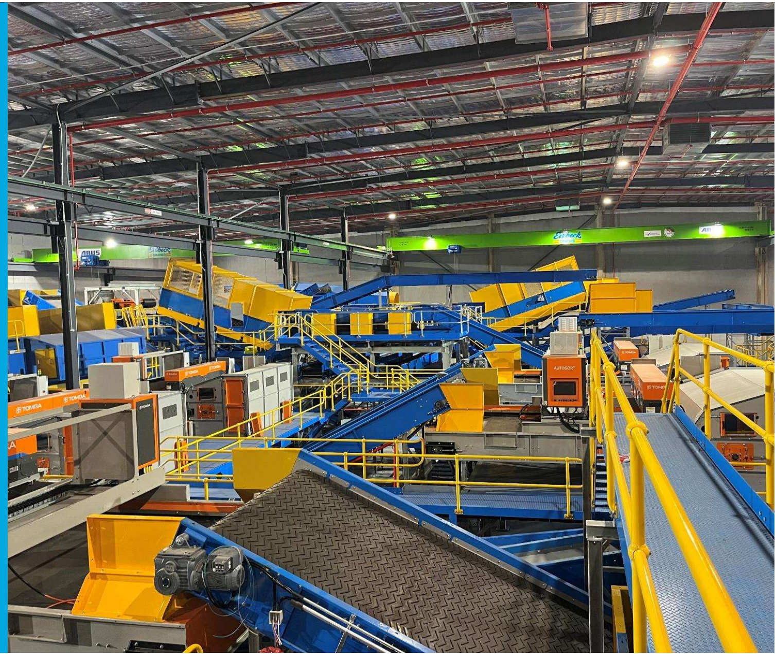
Pictured: Inside Western Sydney MRF pre-commissioning
