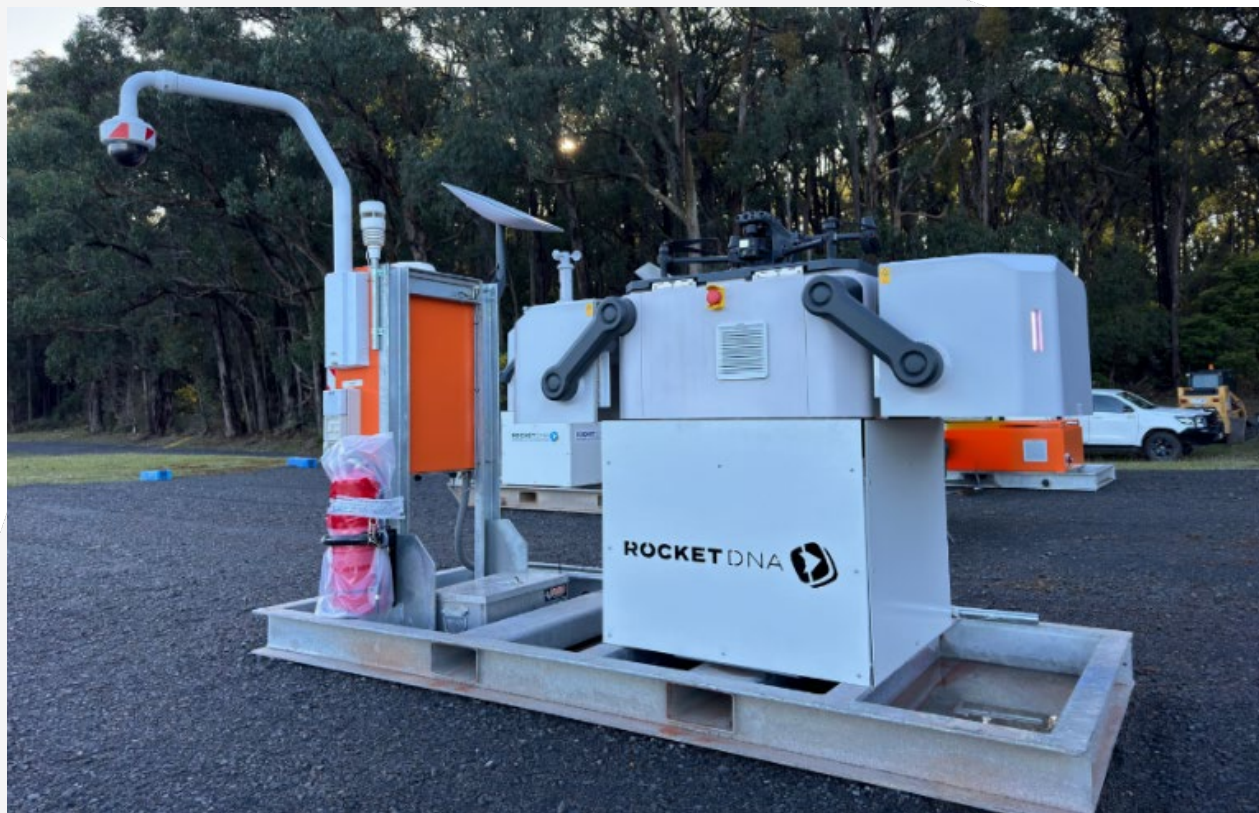
Figure 3: Example of RocketDNA PatrolBot® surveillance solution, installed in Australia
