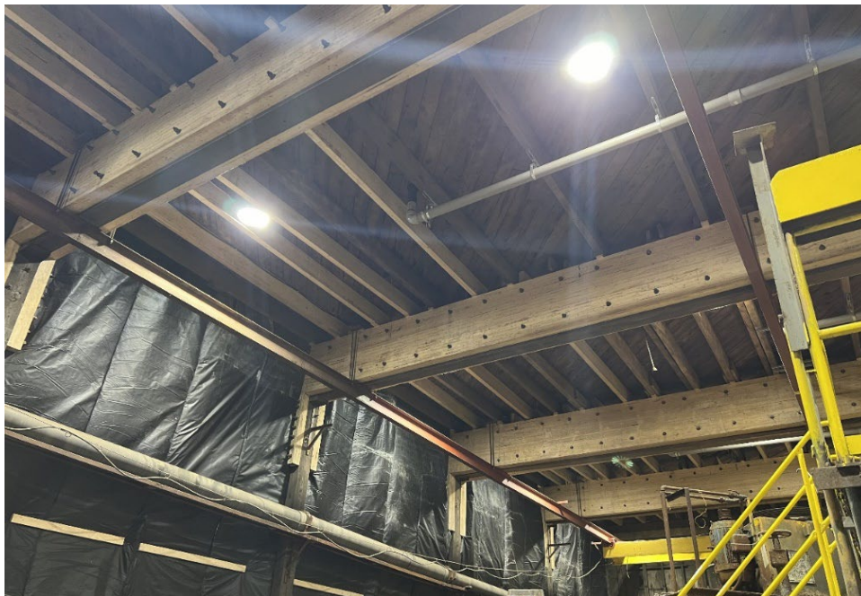
Figure 2: View of the newly replaced processing facility roof through investment by Doré. The entire processing facility is housed within an enclosed industrial-scale shed.
